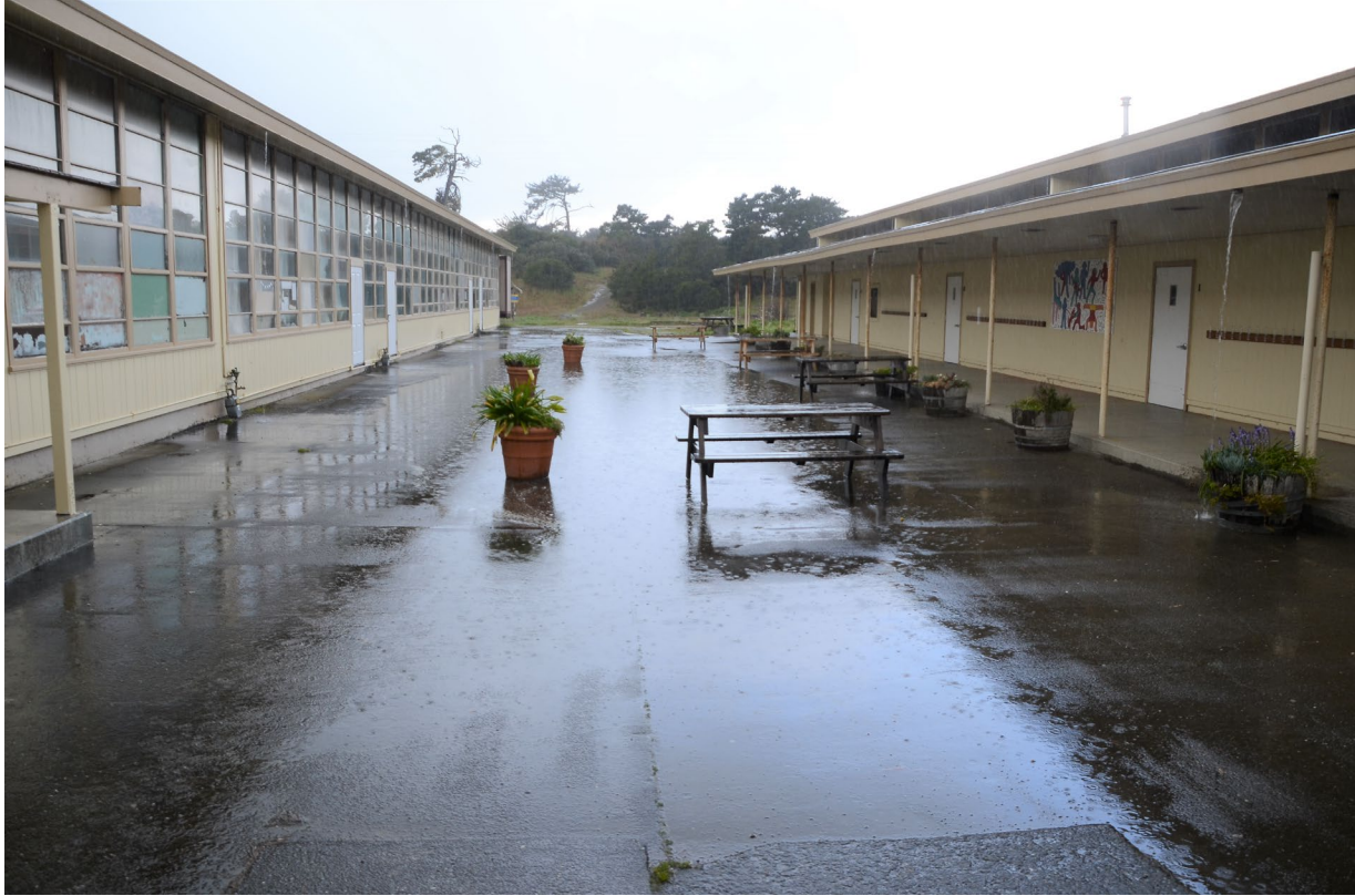
Figure 3. Flooding of the courtyard at the Manila Community Center, occupied by a local charter school. The proposed project will replace the concrete slab with a rain garden.
