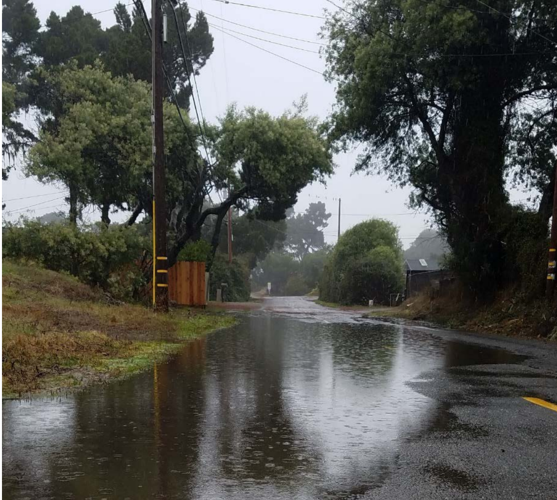
Figure 2. Common Flooding on Peninsula Drive due to Lack of Drainage Infrastructure. The proposed project includes a catch basin and culvert to a bioswale in this location.
